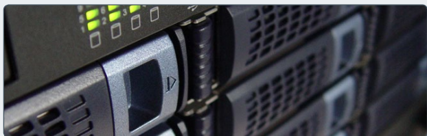
Computer units (UPS)
