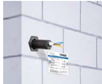
Wall feed-through in sand-lime brick fire-protection wall.
