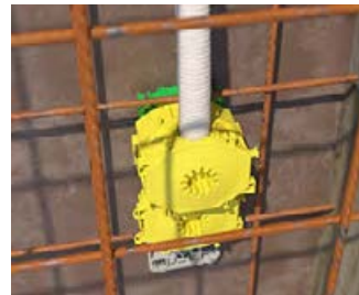
Latch the rear part with conduit onto the front part, then pour concrete.
