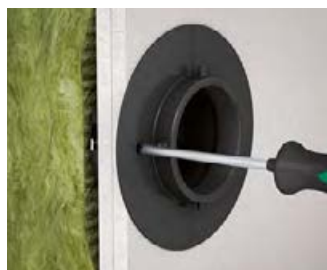
Fix sealing cylinder by tightening the screws (same procedure as with cavity wall boxes).
