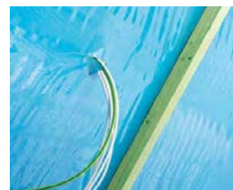
The cables are fed through the building's air-tight seal. This entry must be permanently sealed air-tight.
