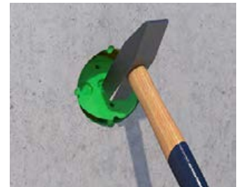
Open the concrete construction boxes or casings, then install the accessories or covers.
