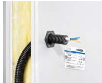
M16 - M25 wall entry, in plasterboard fire-protection wall with M25 conduit.
