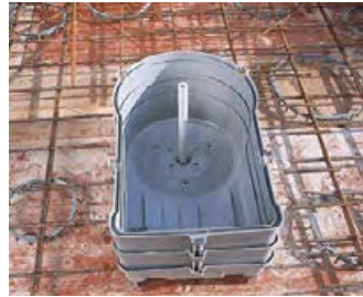
Attach the housing with 2 intermediate frames and a support conduit to the formwork.
