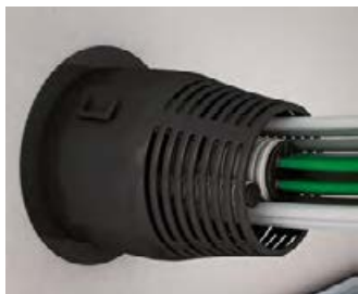
Mixed population of sheathed cables and conduits.
