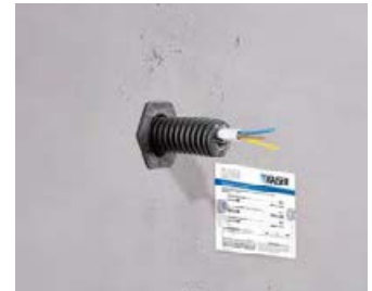
Wall feed-through in concrete fire-protection wall.
