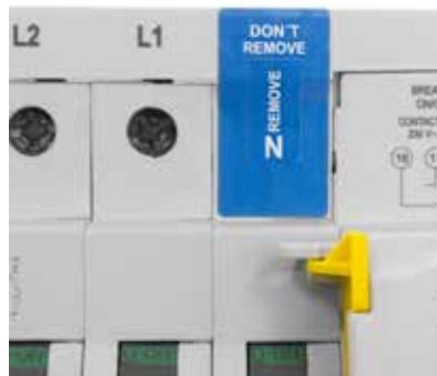
Figure 2: Safety seal on the neutral terminal.
